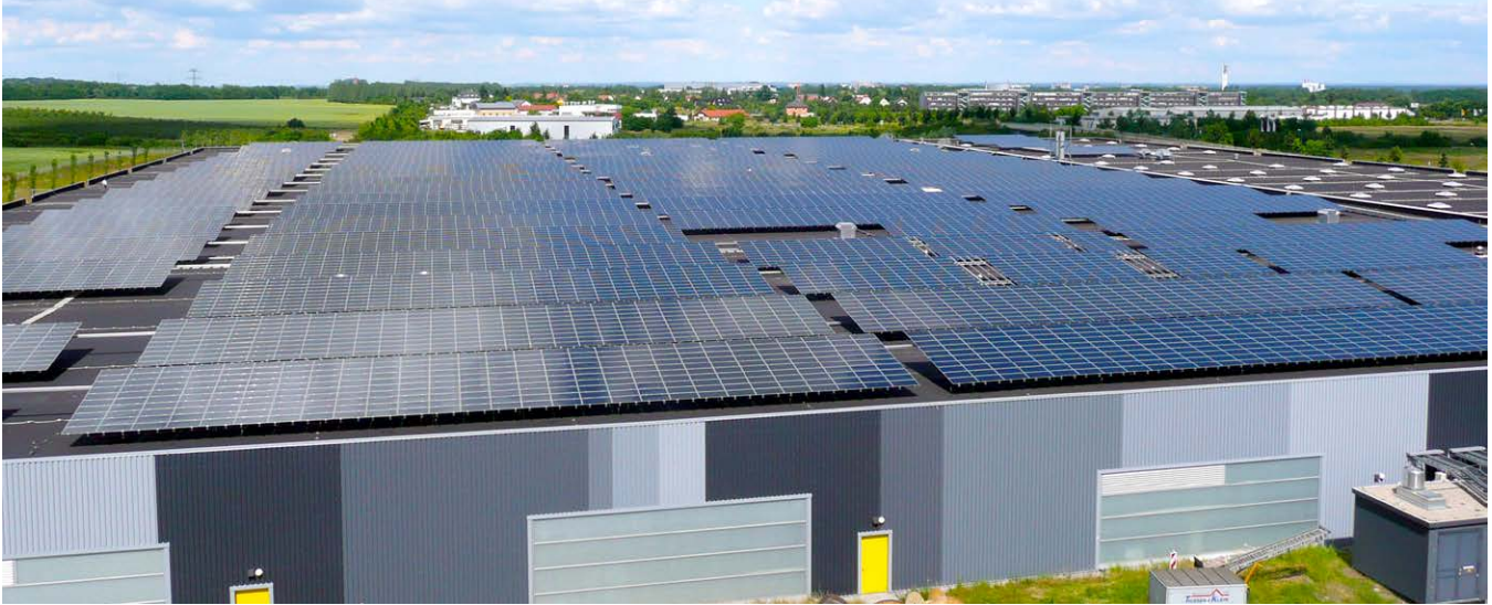
2.9 MW Rooftop PV Installation at First Solar's Recycling Facility in Frankfurt Oder, Germany.
