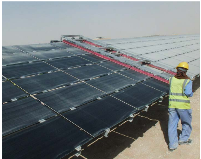
First Solar Manual Dry Brush Trolley at the 13MW DEWA solar PV power plant in Seih Al Dahal, United Arab Emirates
